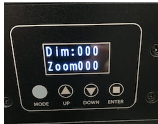
NO DMX CABLE CONNECTED
